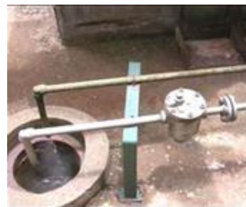
倒筒式祛水器排水洩漏
